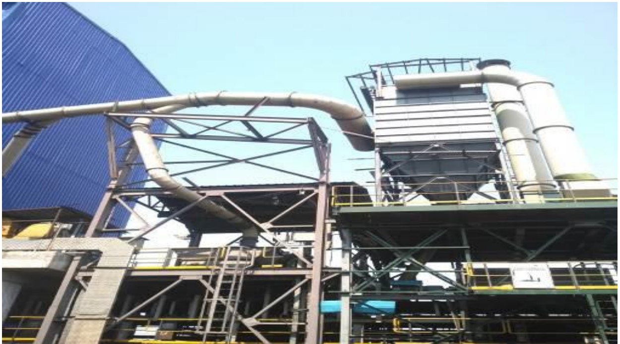
DUST EXTRACTION SYSTEM AT TRANSFER POINTS
